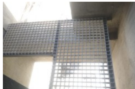
Plumbing Duct Platform
